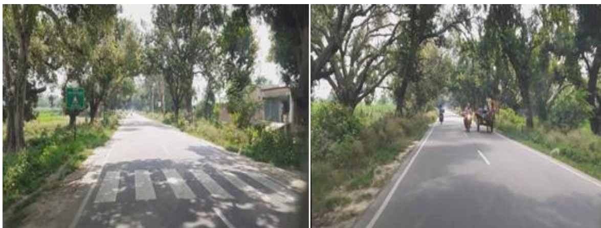
Figure 1.4: Present Road Condition
